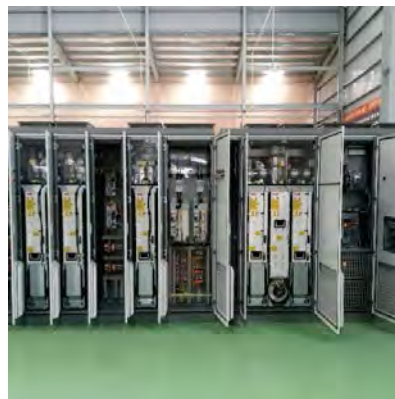
Motor control center
